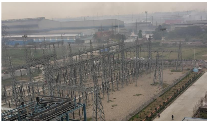
Exhibit 1: STL's captive 220kV sub-station
